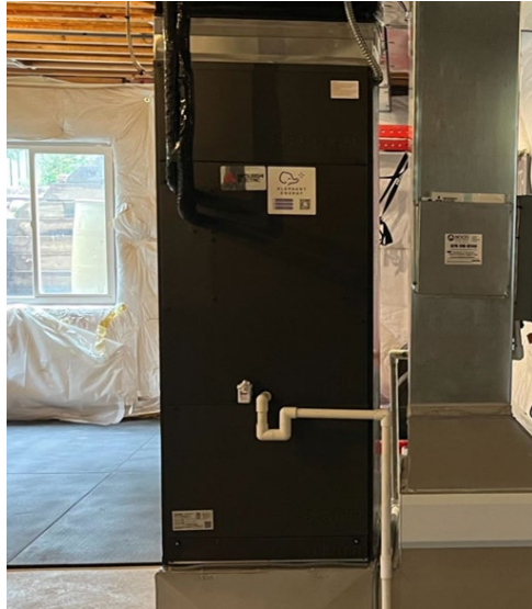
Indoor Air Handler Unit
