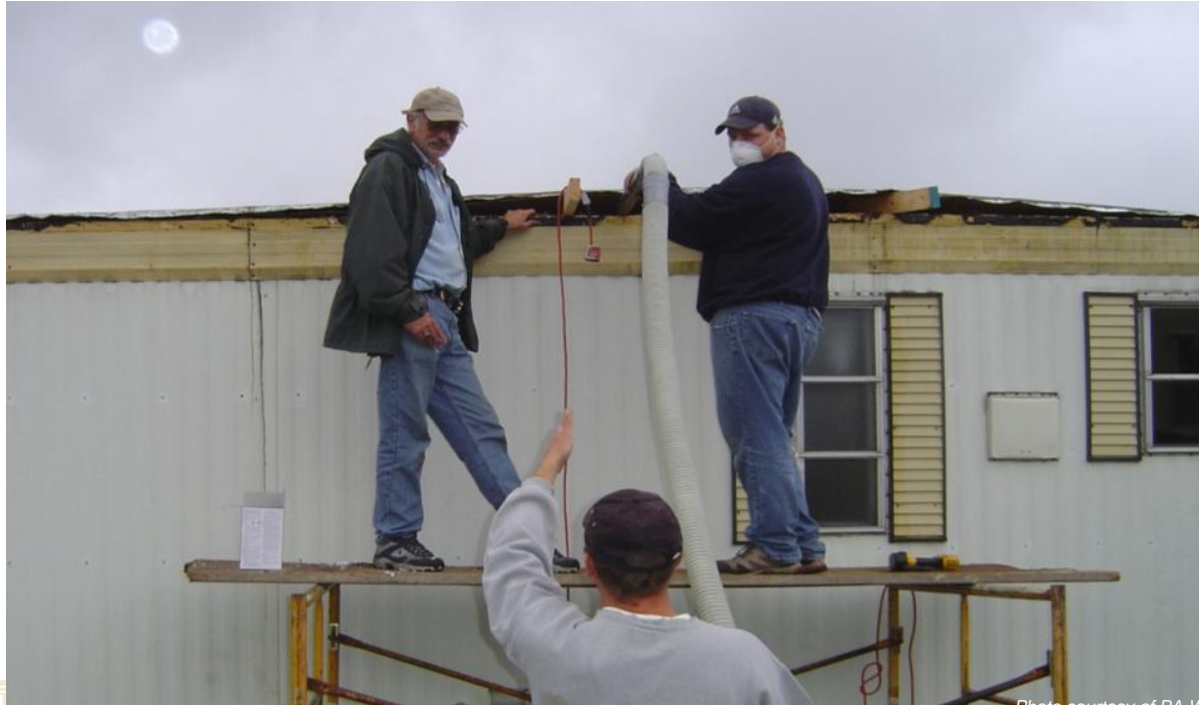
Photo courtesy of PA W
