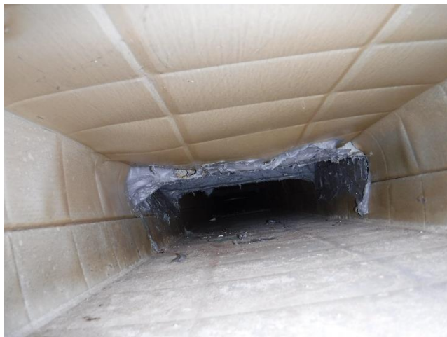
Riser to Trunk
