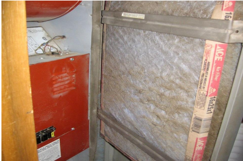
Return Front of Furnace
