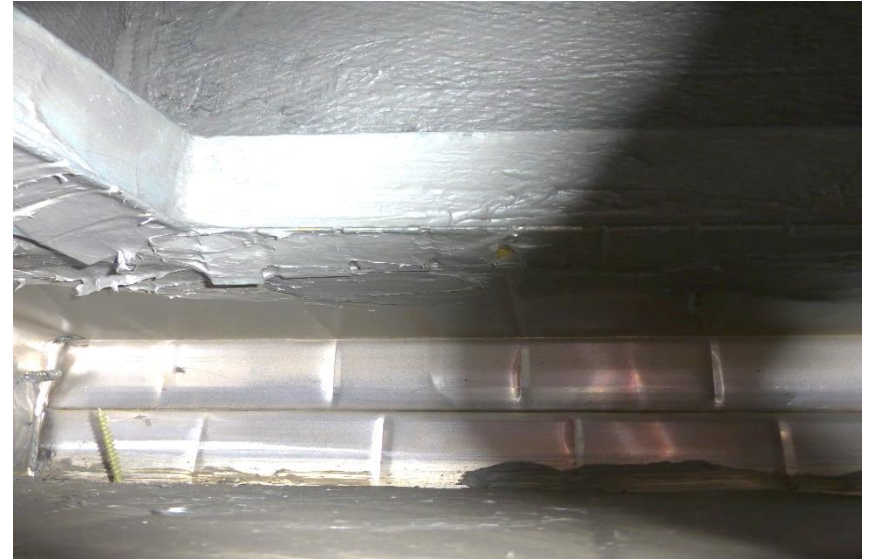
Plenum View from Below
