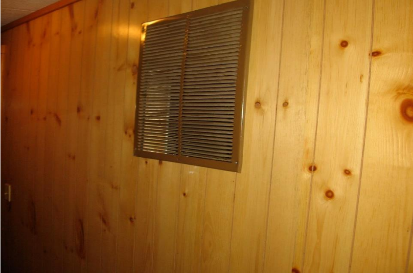
Return air path/ grille wall
