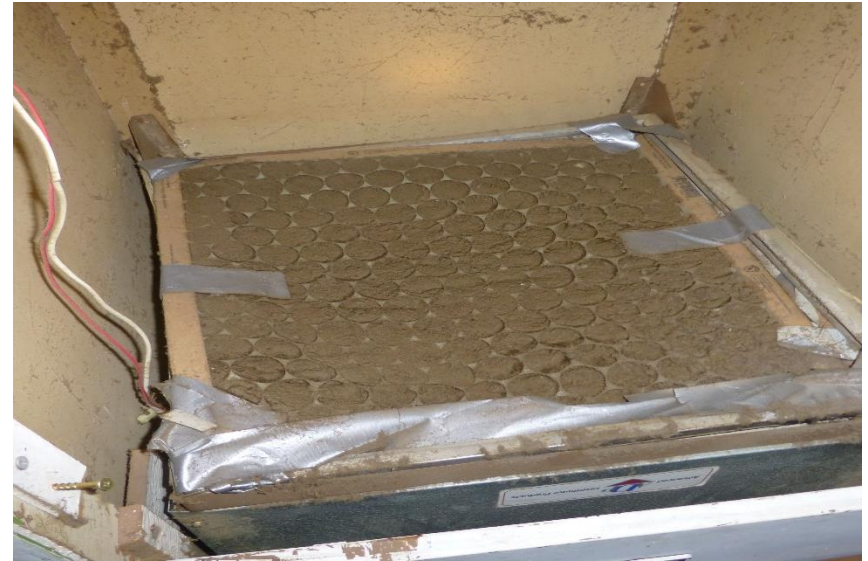
Return Top of Furnace
