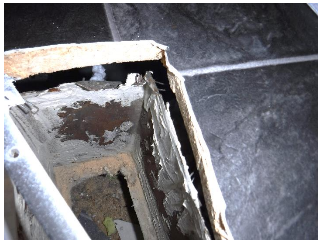
Riser to floor
